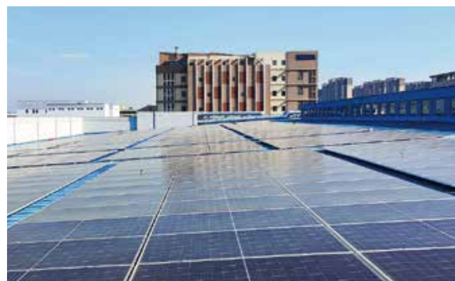
1.8MW ↻ Industrial and commercial rooftop projects Wuxi, China
