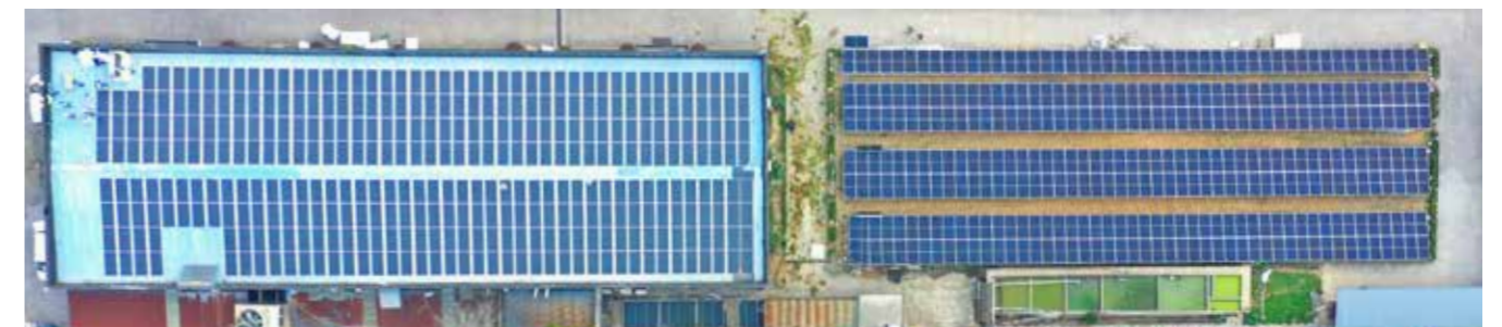
800KW ↻ Yifeng Distributed Photovoltaic Project Yangzhou, China
