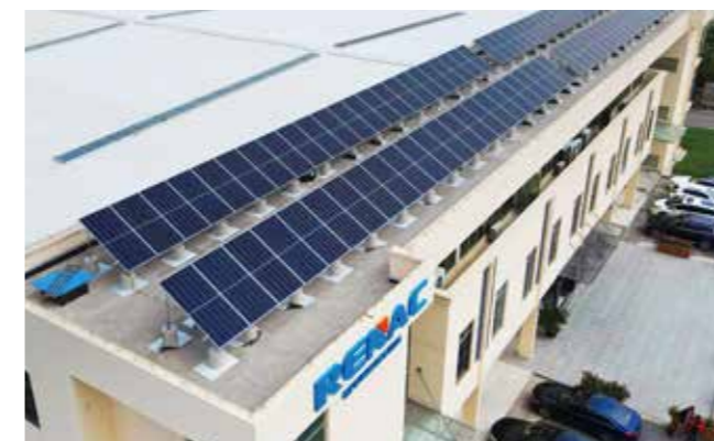
55KW ↻ Natong Optical storage and Charging project Suzhou, China
