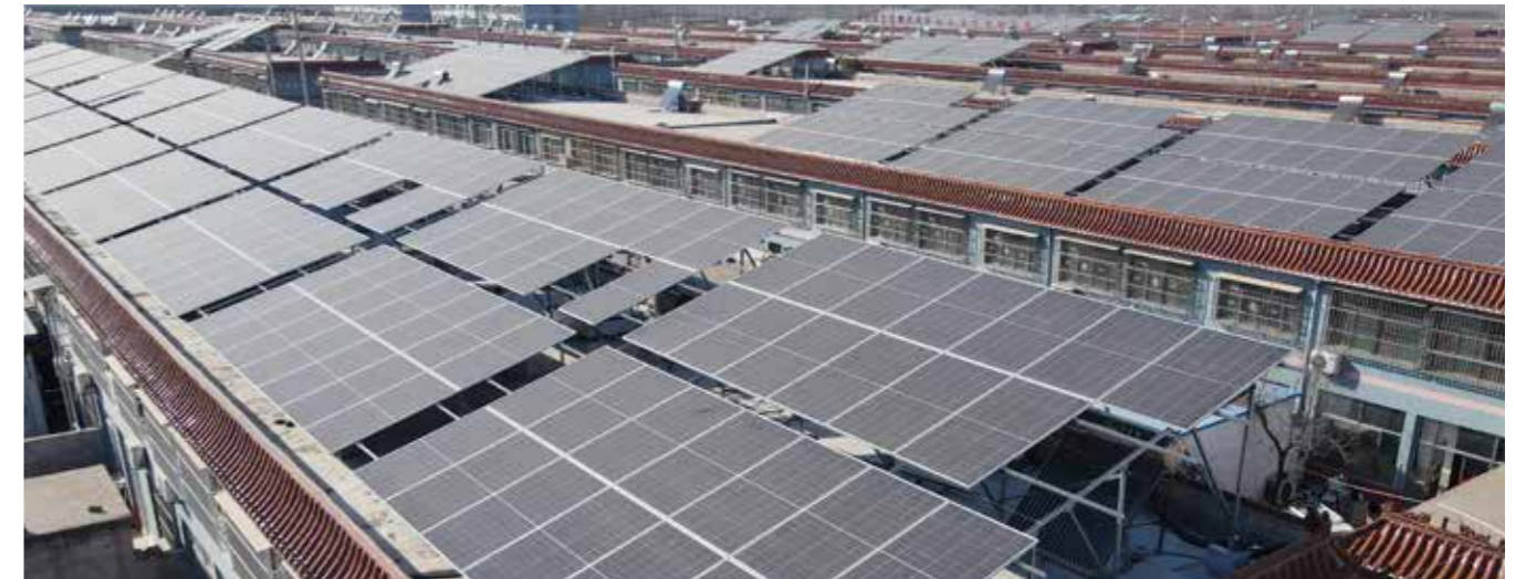
5.5MW ↻ Liaocheng Roof Top project Shandong, China
