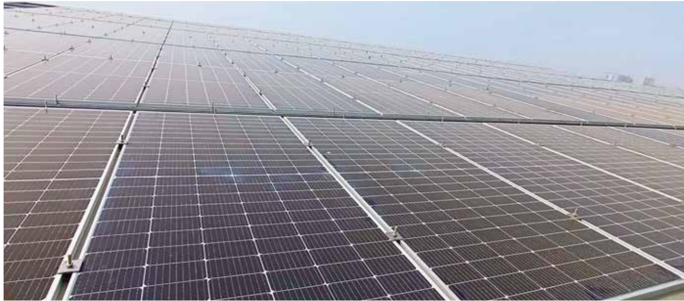
93.6KWP 📍 Swimming pool shed with Solar
