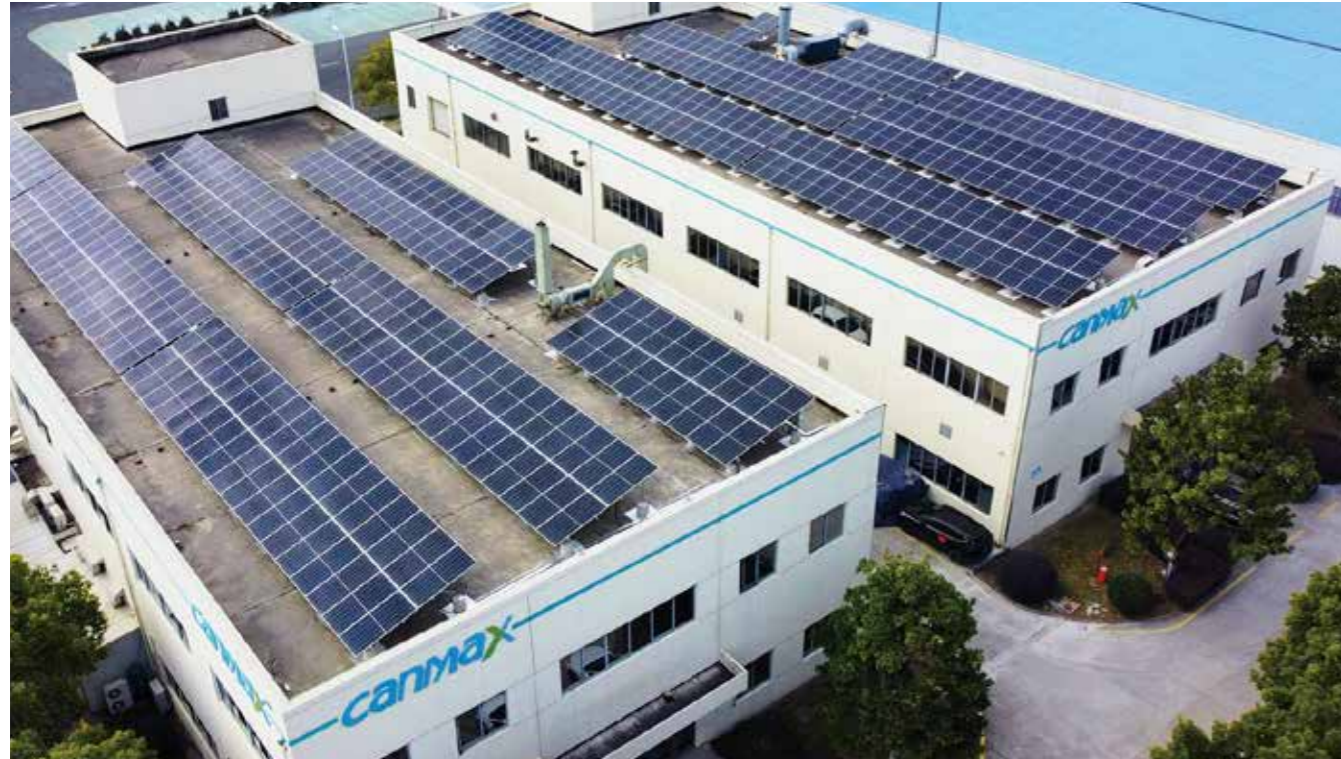
1MW ↻ Tianhua Industrial and Commercial Roof Project Suzhou, China
