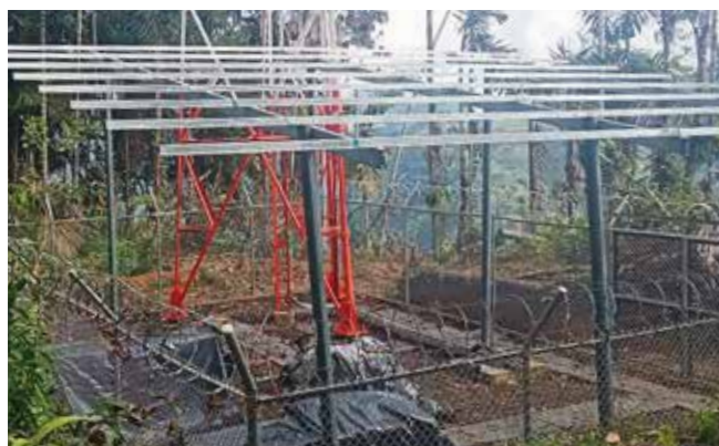
200 SETS 📍📍 Ground Mounted Solar Power Lenercom - Colombia
