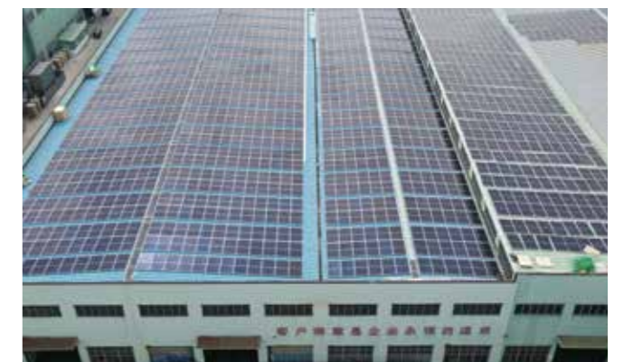
6MW ↻ Distributed Photovoltaic Project Yixing, China
